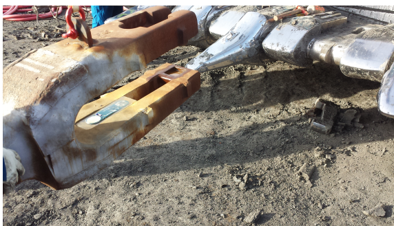
Figure 4.23: The sensor node inside the adapter while it is lifted and being attached to the bucket on an operational shovel.
