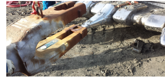
Fig. 7. The SeN inside the adapter while it is lifted and being attached to the bucket on an operational shovel.
